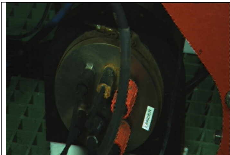
Figure 18. Photo of end cap on optical comms pressure housing showing corrosion around bulkhead connector
