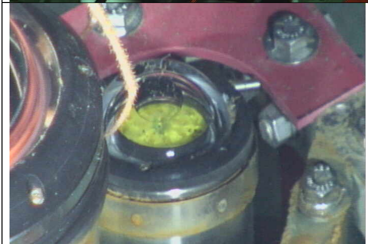
Figure 19. Photo showing a bubble in the emitter pressure housing indicating a leak.
